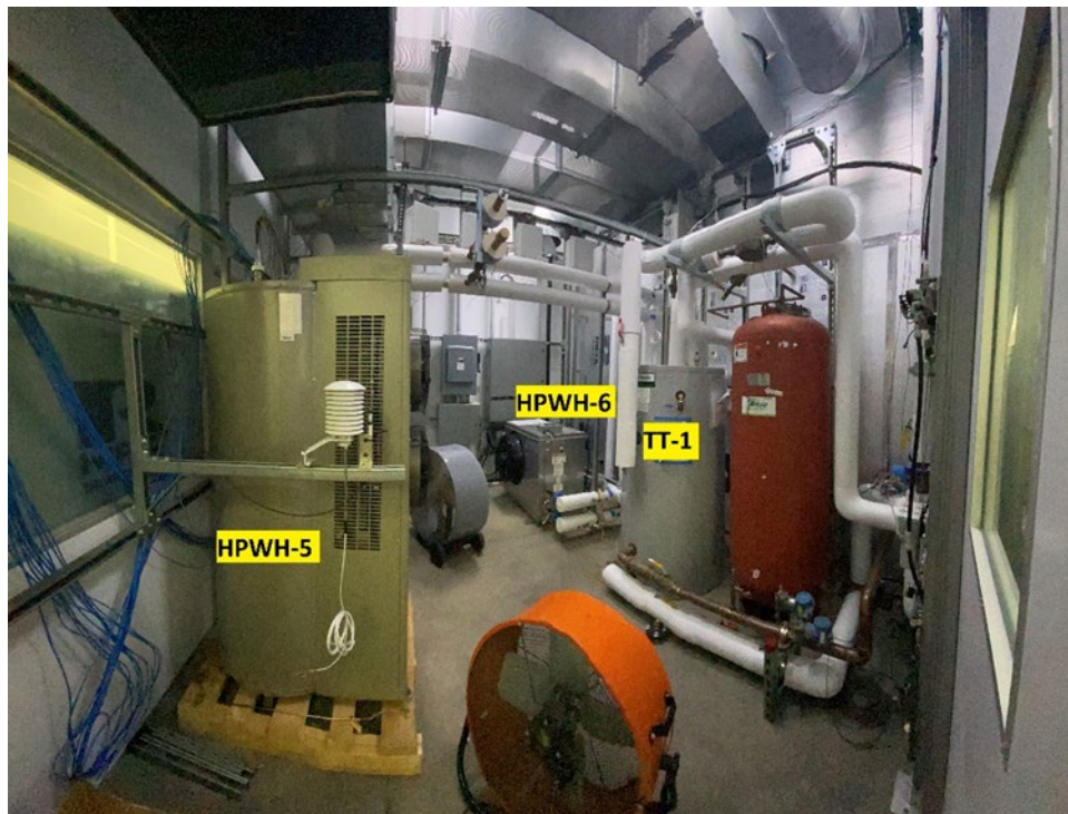
Figure 10. East chamber equipment placement.
