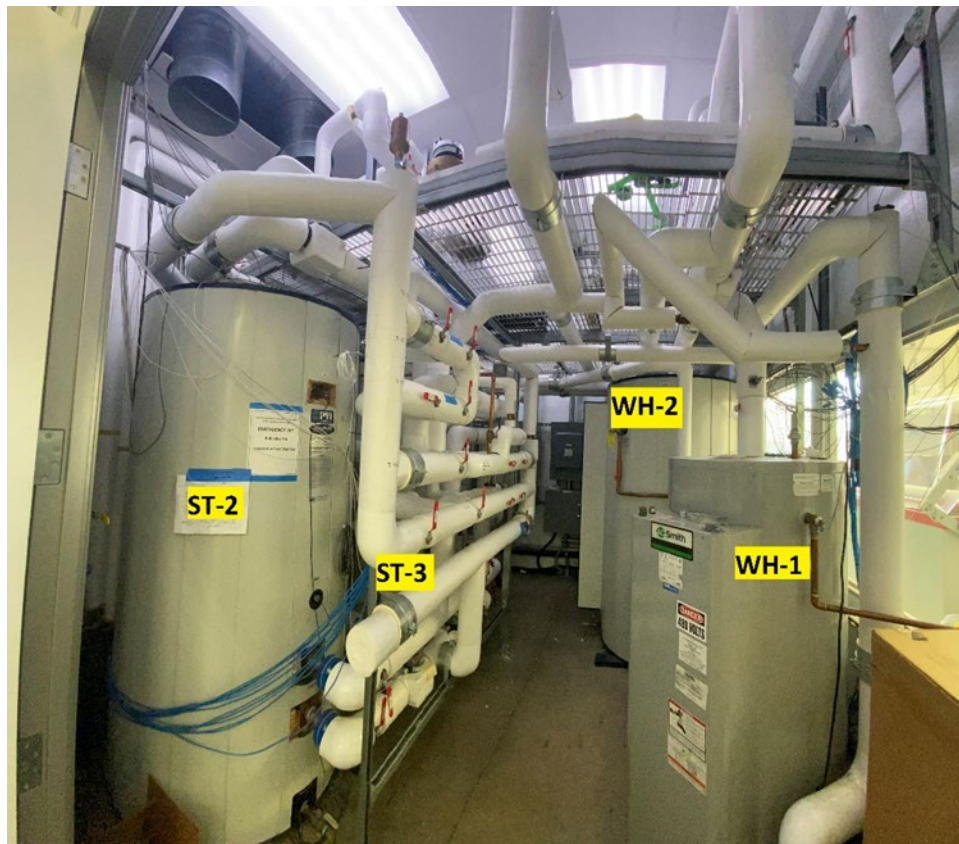
Figure 9. West chamber equipment placement.
