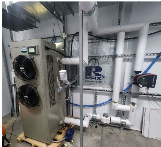
Figure 6. AO Smith CHP-120 as installed for testing.
