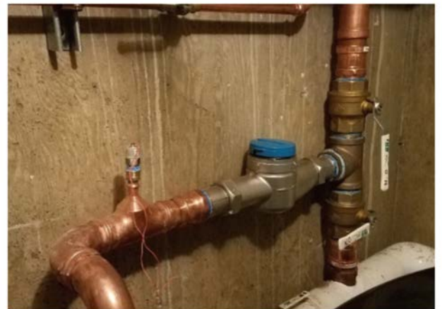
Figure 7. M&V Temperature Sensor and Flow
