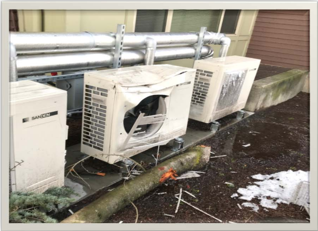
Figure 8. Snowstorm and Tree Damage to CU-3.
