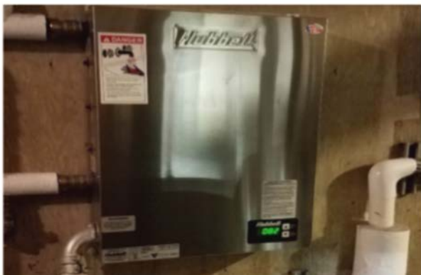
Figure 6. Instantaneous Electric Water Heater (Existing EB-1)
