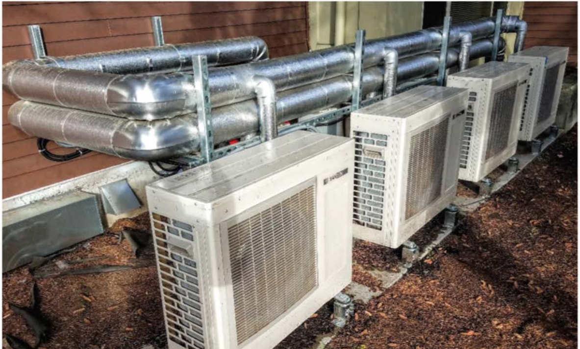
Figure 2. Sanden HPWHs After Pipe Insulation (CU-1, 2, 3 and 4)
