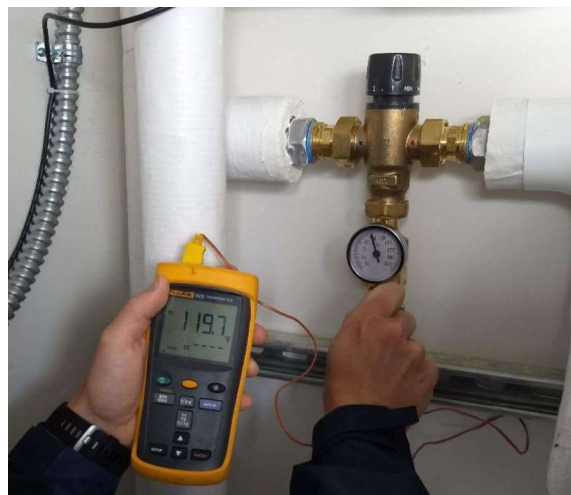
Figure 3. Thermostatic mixing valve with water temperature outlet of approximately 120°F.
