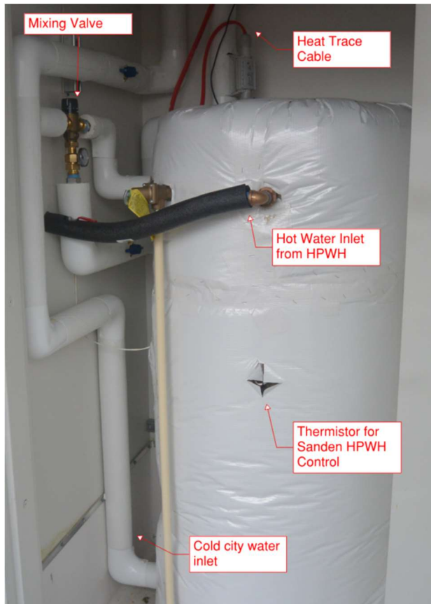
Figure 2. Hot water storage tank on Level 4
