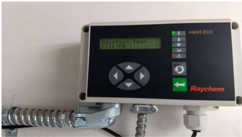
Figure 4. Temperature maintenance heat trace set to maintain 116°F in distribution piping.
