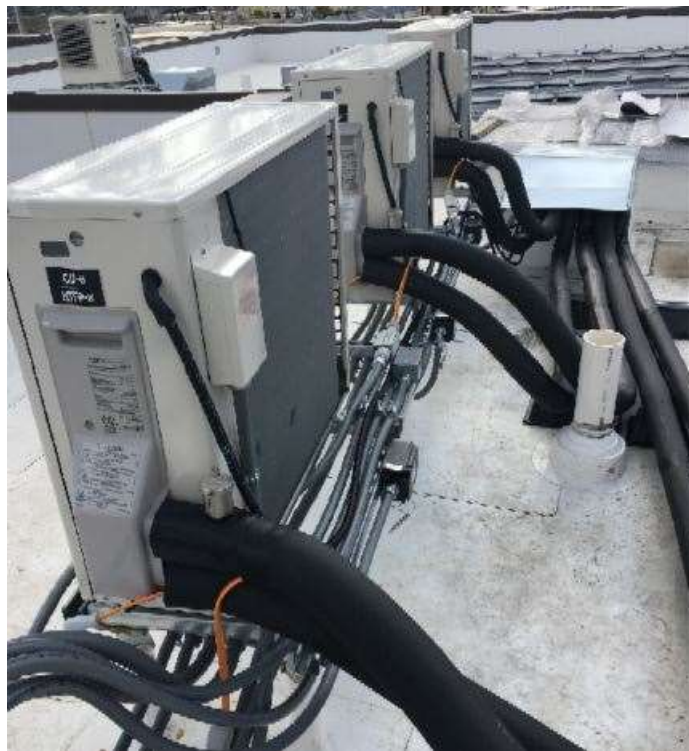
Figure 5. Rooftop Sanden HPWHs with freeze protection heat trace.
