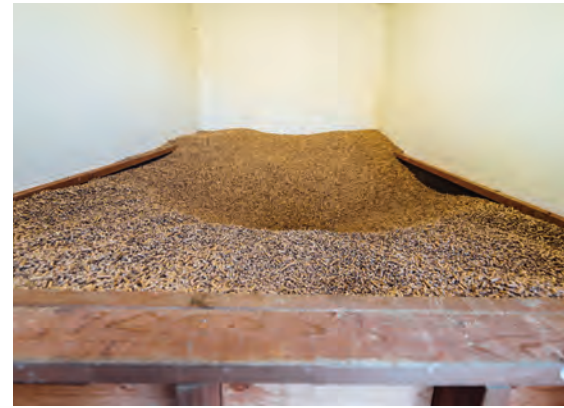
Pellets for the pellet boiler are manually loaded into the storage hopper (shown here) and transported by an auger mechanism into the pellet boiler's burn chamber.
