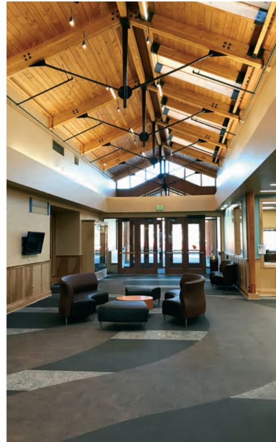
Harrigan Centennial Hall's heating and cooling is provided with a zonal air-to-air VRF heat pump with ductless ceiling cassettes in most zones.
