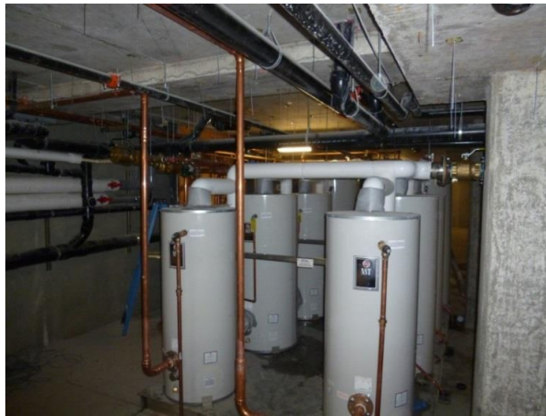
Figure 4: Stream Uptown Hot Water Storage Tanks on two sides.
