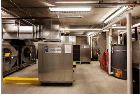
Figure 3: Colmac Industries RCC Equipment
