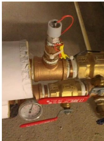
Figure 10: Hot water temperature sensor
