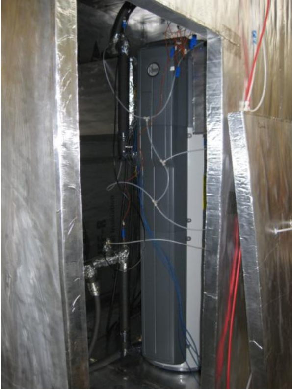
Figure 2. EcoSense Installed in Test Chamber
