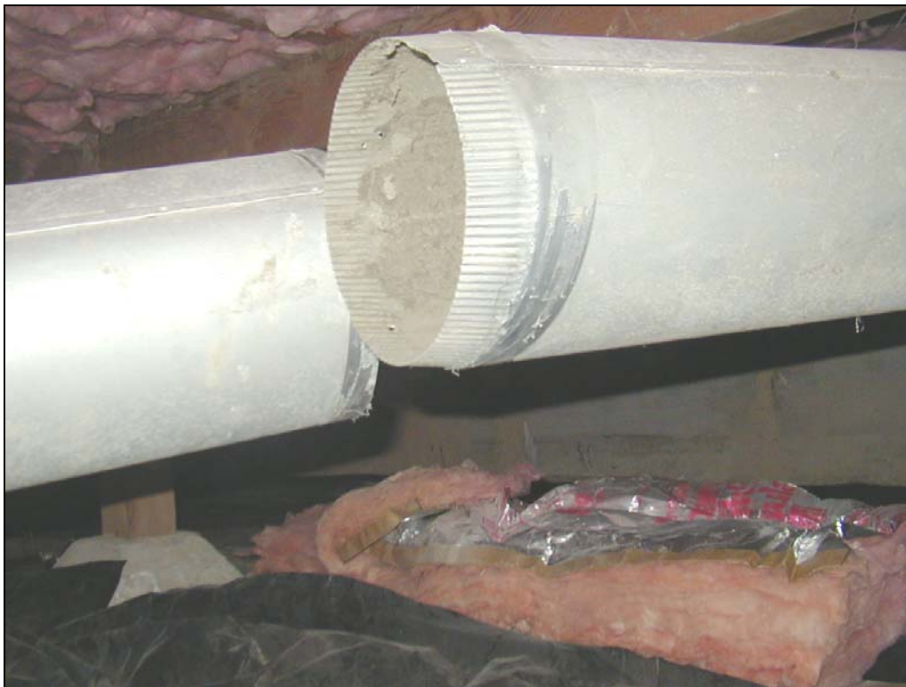
Figure E4. Added return leak in return duct.
