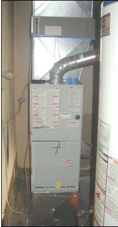
Figure H2. Downflow gas furnace in garage.
