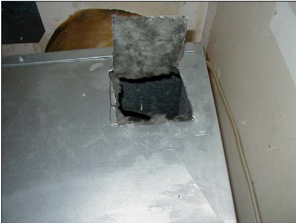
Figure A4. Added return leak at plenum.
