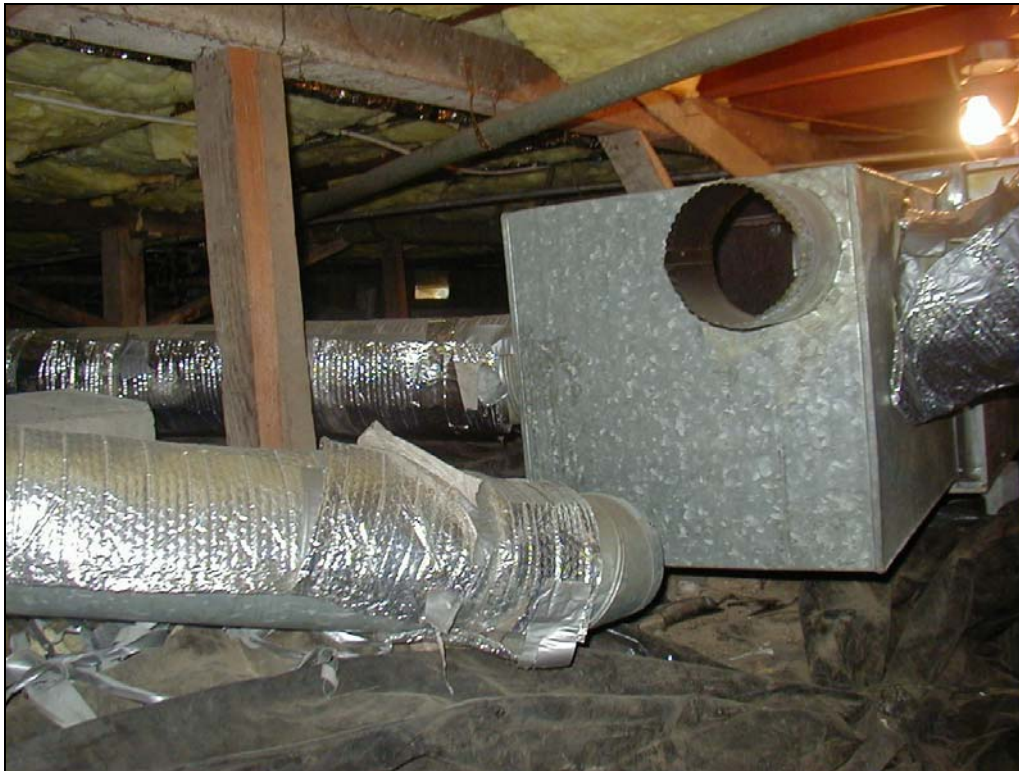
Figure F3. Added supply leak at plenum.
