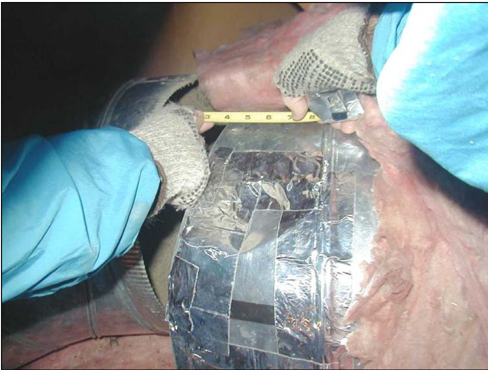
Figure C4. Added leak in return duct.
