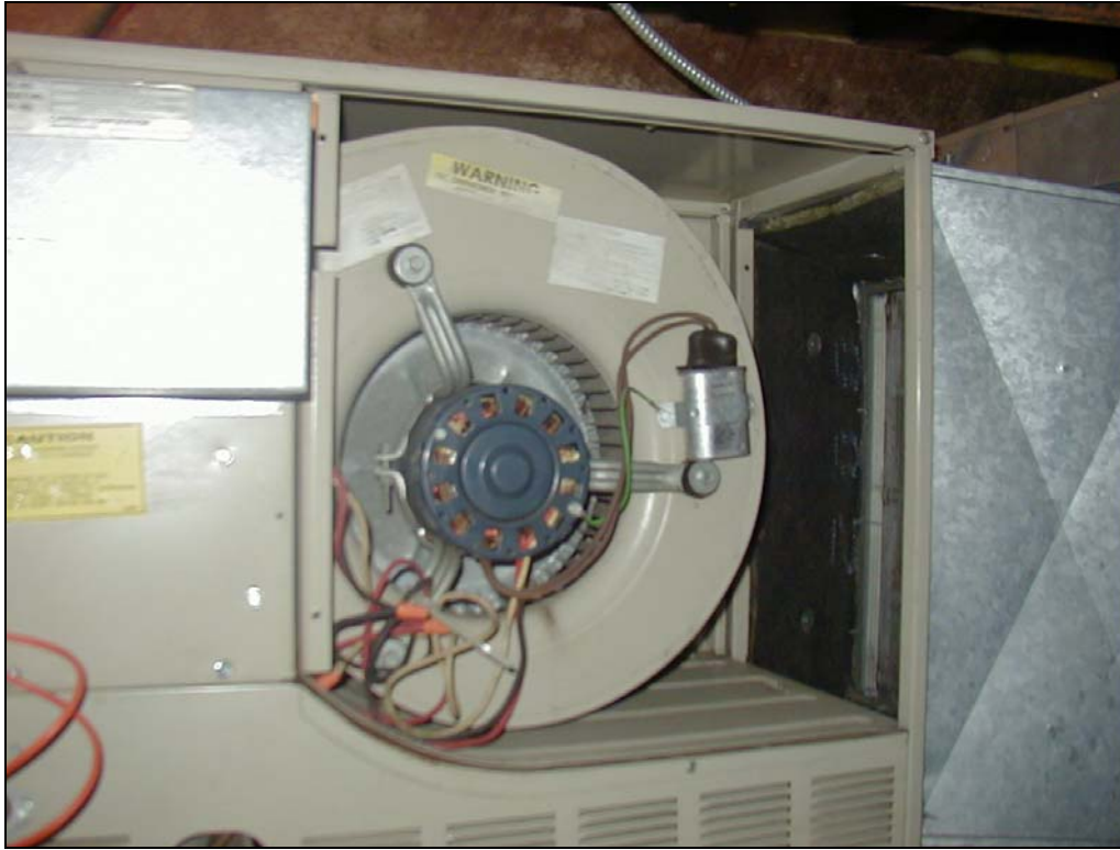
Figure F2. Horizontal gas furnace in crawl space.
