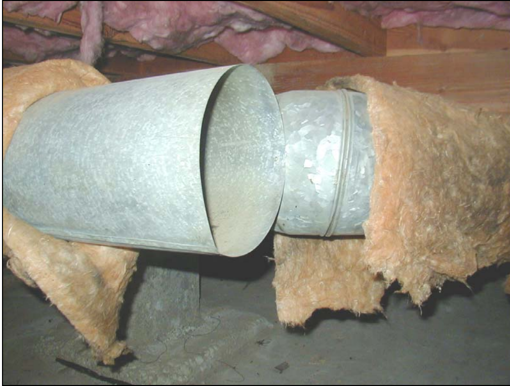
Figure H5. Added supply leak in trunk.
