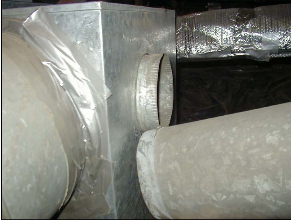
Figure F4. Added return leak at plenum.
