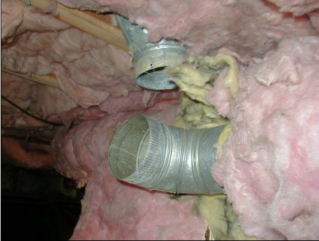
Figure D2. Added supply leak at register boot.
