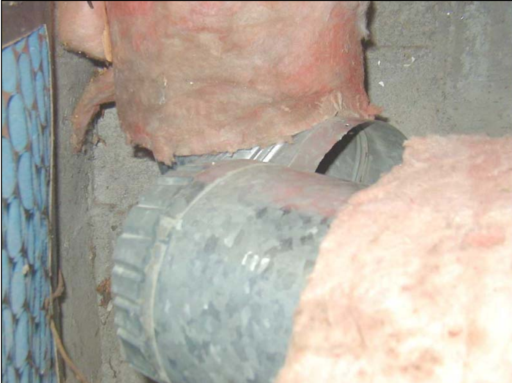
Figure I3. Added supply leak at register boot.
