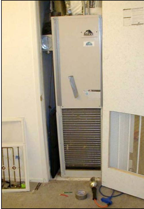
Figure G2. Downflow heat pump in closet in conditioned space.
