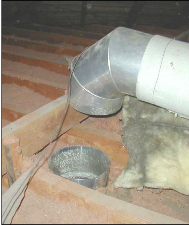
Figure E3. Added supply leak at register boot.
