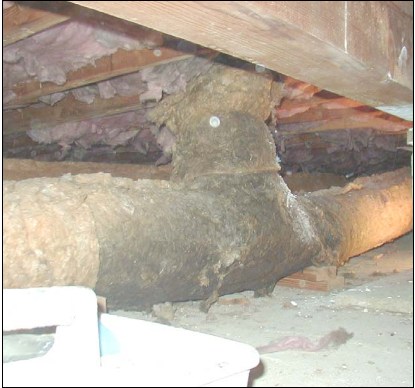
Figure H3. As-found leak in supply trunk (dirtier insulation indicates larger leakage).
