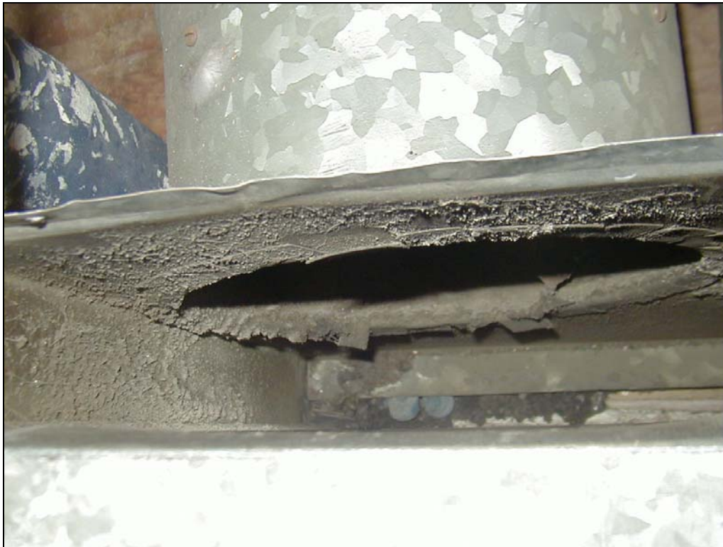
Figure H4. One of the as-found return leaks at junction box (note fingers).
