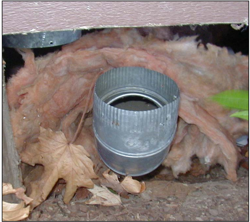
Figure C3. Added supply leak at register boot.
