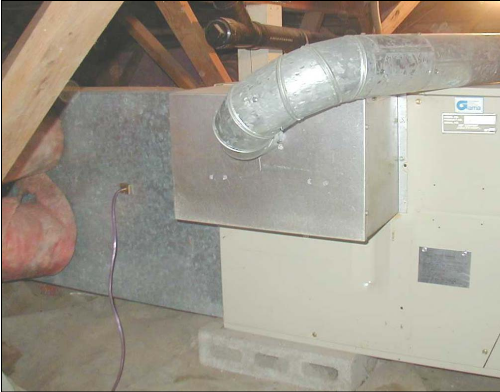
Figure I2. Horizontal gas furnace in crawl space.
