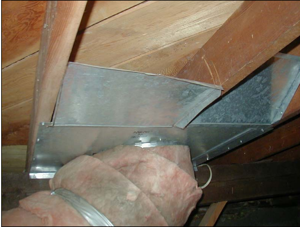
Figure I4. Added return leak at panned joist at grille.
