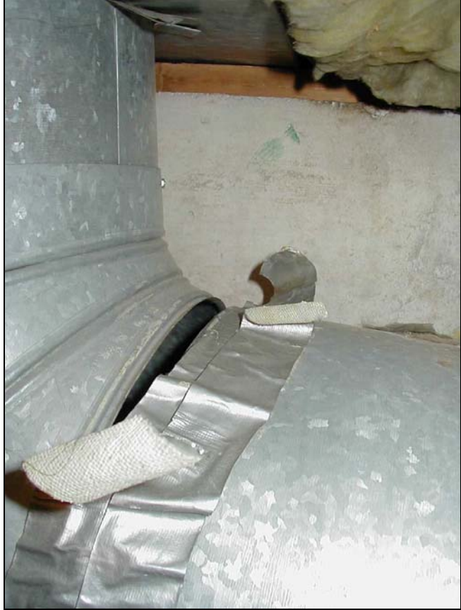
Figure A3. As-found leak in supply trunk.
