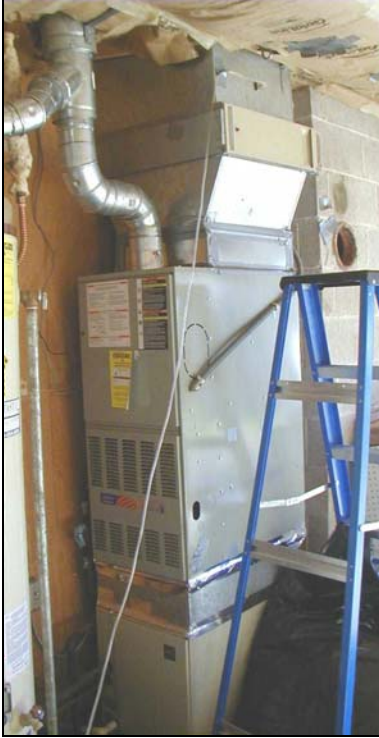
Figure C2. Downflow gas furnace in garage.
