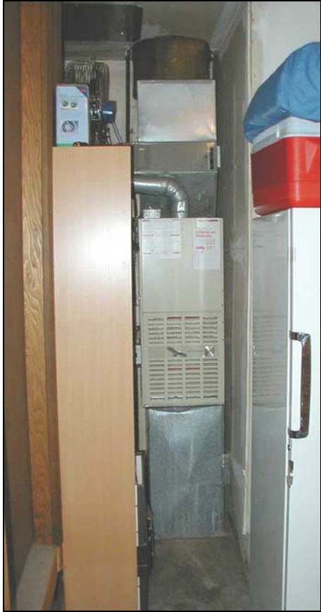
Figure A2. Downflow gas furnace in garage.
