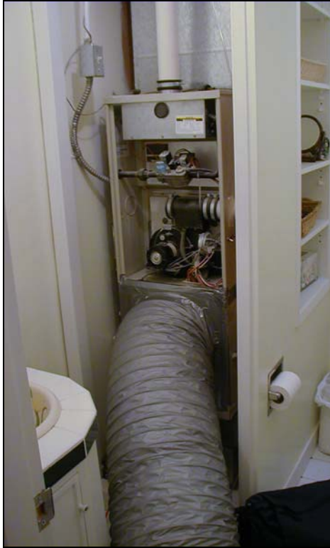
Figure E2. Upflow gas furnace in closet.
