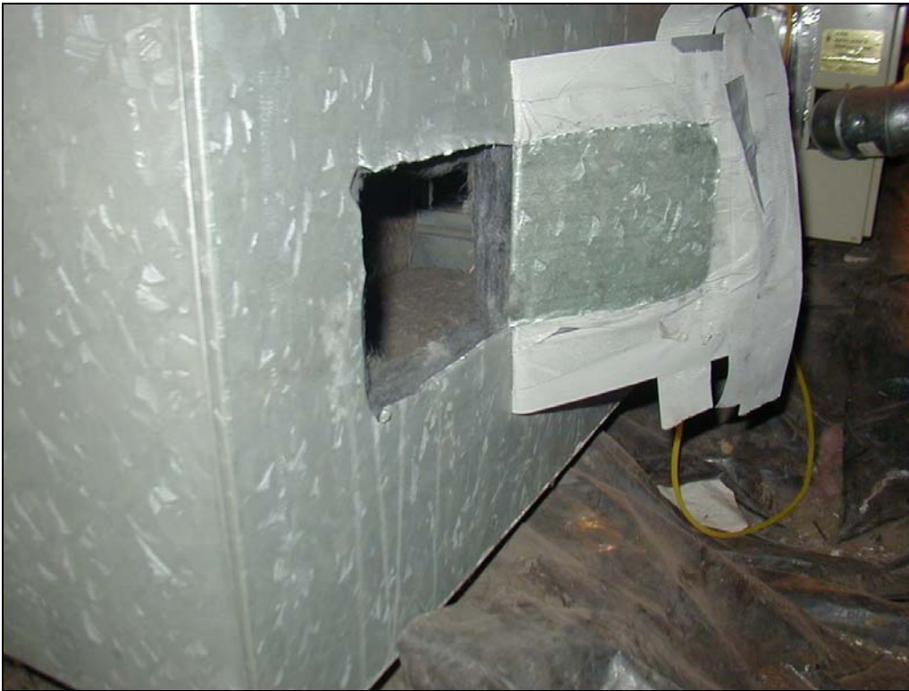
Figure D3. Added return leak at plenum.
